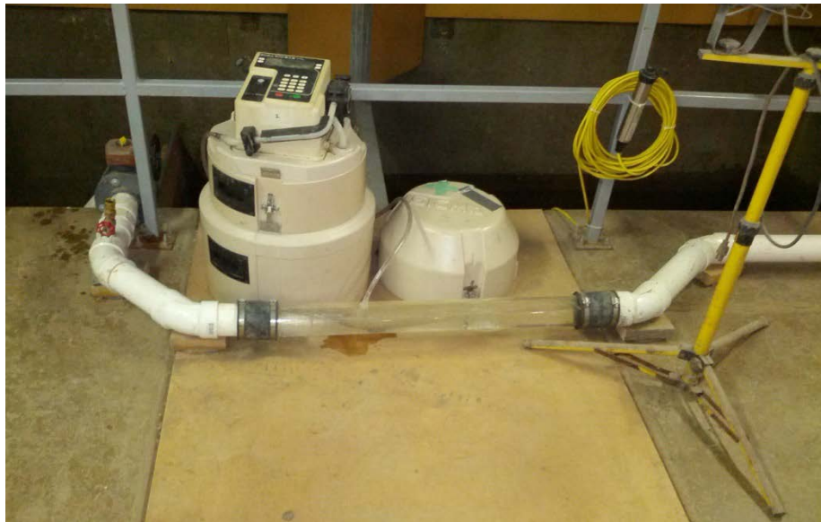
Figure 3.6. SIGMA automated sampler and pressure transducer near outlet pipe
